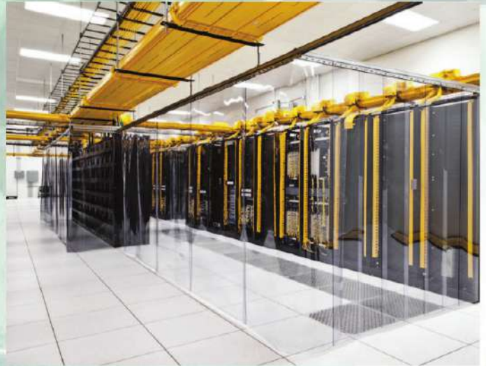
CONTAINMENT DATA CENTER
