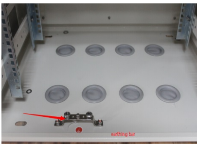
Copper Earthing Bar
