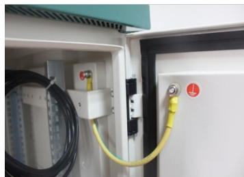
Copper Earthing Bar
